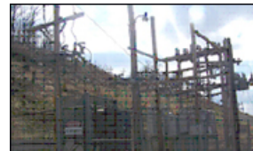
Electric utility substation
